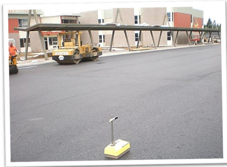
Columbia West conducting pavement testing and evaluation at Grass Valley Elementary School.
