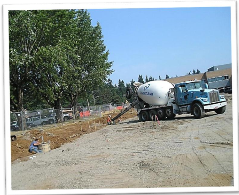
Columbia West testing concrete at Helen Baller Elementary School in Camas, Washington.
