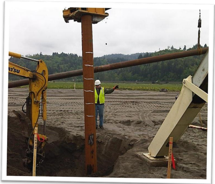
Columbia West conducting steel pile testing and inspection at the OALC Church in Woodland, Washington.
